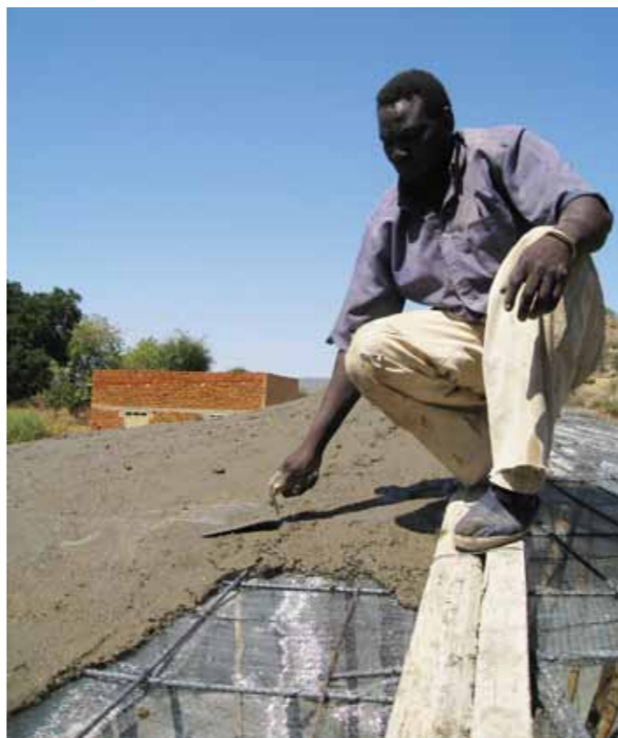
A FAR-trained mason constructs a cement tank for a rooftop water catchment in South Kordofan
